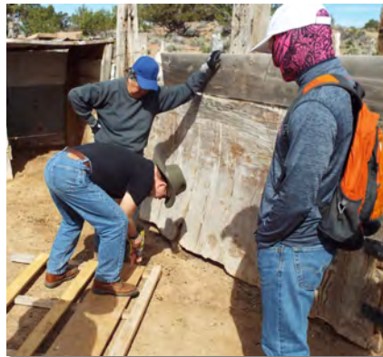
Mission volunteers help a member of the parish repair the gates at her sheep corral.
