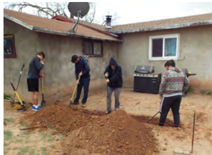
Volunteers learn by doing, including digging a foundation trench for an addition to this parishioner's house.
