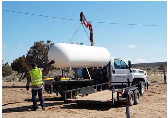
Workers from Nations Gas Technologies unload the Mission's new 1,000 gallon propane tank.
