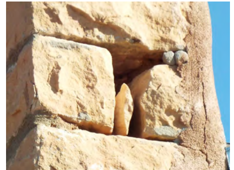
Loose stones on the Mission church facade prior to the repointing work.
